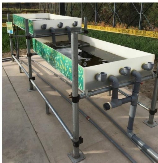
Figure 5 The INNOQUA BSP, as installed after the lumbrifilter at the demonstration site in Peru
