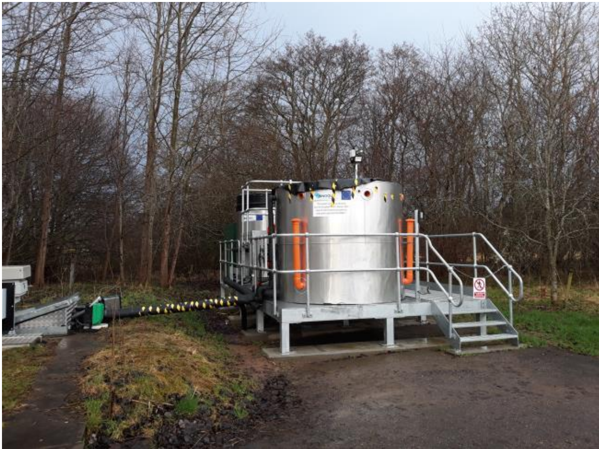
Figure 2-1 INNOQUA Installation at Littlemill, Scotland
