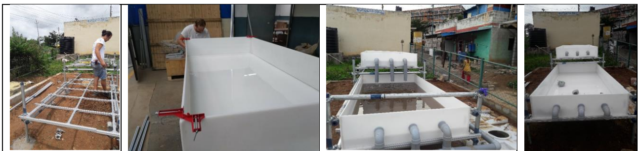
Figure 3-5 India on site manufacturing of the BSP module by the INNOQUA project team
